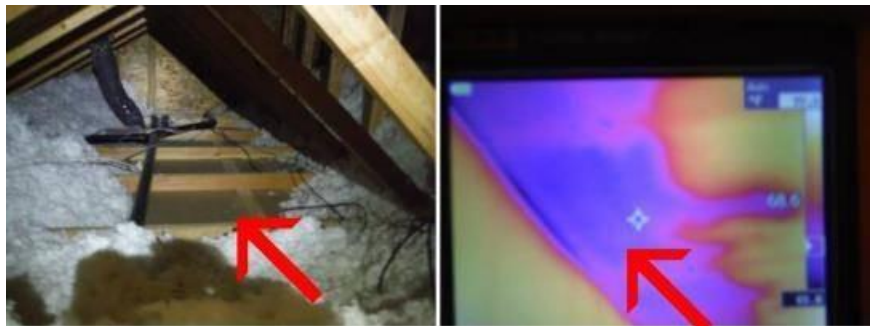
Insulation over the NE bathroom has been moved for some repairs and not replaced. This is visible in the attic and with a thermal camera, recommend repairs and adding additional insulation if needed.
