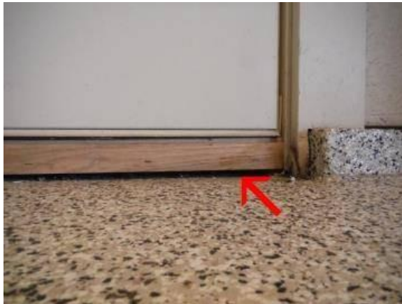
Gap is visible under the threshold on the outside entry door to the garage, with evidence of past water entry. Recommend sealing.
