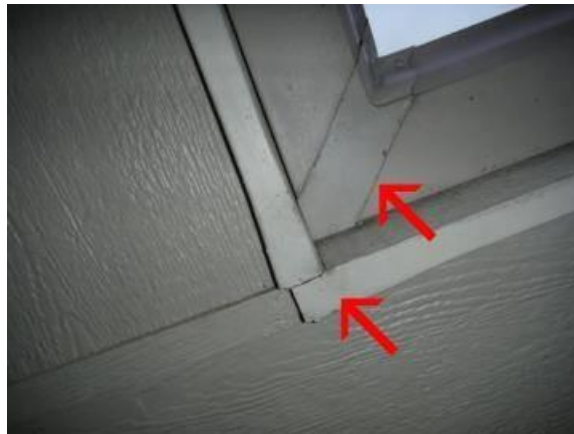
Evidence of leaking is noted at the gutter joints. This can cause damage to fascia. Recommend re-sealing joints and end caps.
