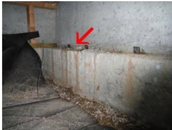
Evidence of past water entry is noted in the crawl space, Ground should slope away from home. Extend gutters away from foundation. Adjust or move sprinklers away from the foundation.
