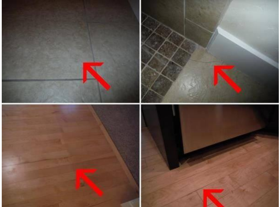
Couple of tiles are cracked at the entry to the master bathroom and one by the shower in the NE bathroom.
