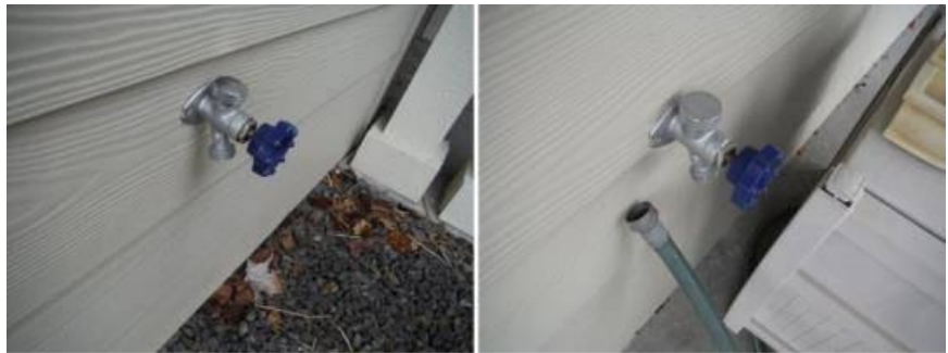
Both of the exterior faucet did not work when tested. Further evaluation and possible repairs needed.
