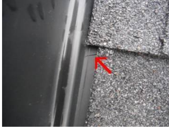
Small crack is visible in the dryer vent cover on the roof, recommend sealing or replacing.
